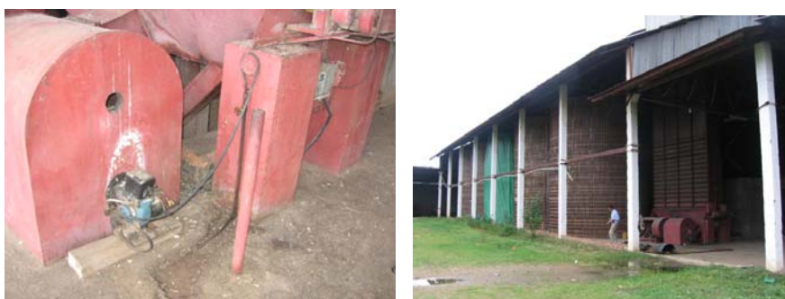
Images of the diesel-powered heating equipment and the silos of the grain drying installation.
